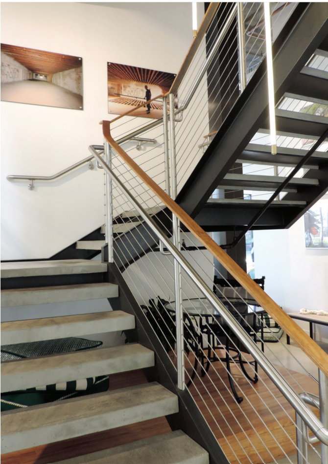
Brown Jordan, maker of innovative outdoor furniture, hired Aim Con Steel to install the stairs and cable staircase railing for its store in the Miami Design District.
