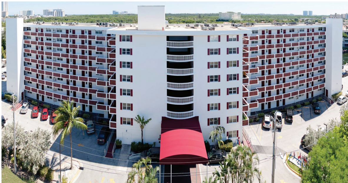
Tru Colors Contracting performed pressure cleaning, concrete restoration and exterior painting services on the Eastern Shores Homeowners Association building, located in North Miami Beach, Florida.
