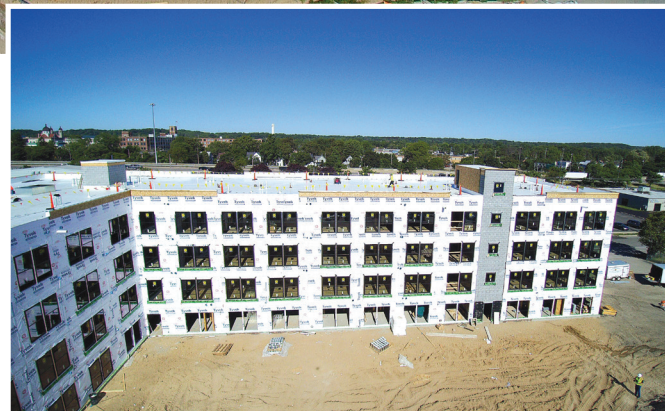
Located in Grand Rapids, Michigan, Grand View Place is a new apartment complex that features spacious one- and two-bedroom apartments. Summit Building Services, LLC framed the four-story, 80,000-square-foot building in 60 days.
