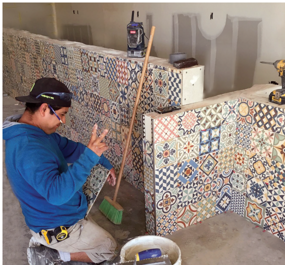
A Handian Construction professional carefully installs decorative Mexican tile at Lola's Mexican Cuisine in Long Beach, Calif.
