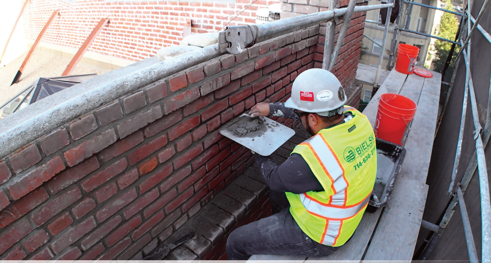
An employee performs tuckpointing on the façade of The Old Soap Factory in San Diego. Tuckpointing is a labor-intensive process of repairing mortar joints in stone or brick masonry walls by grinding or raking out the old mortar to a certain depth, and then refilling with new mortar.
